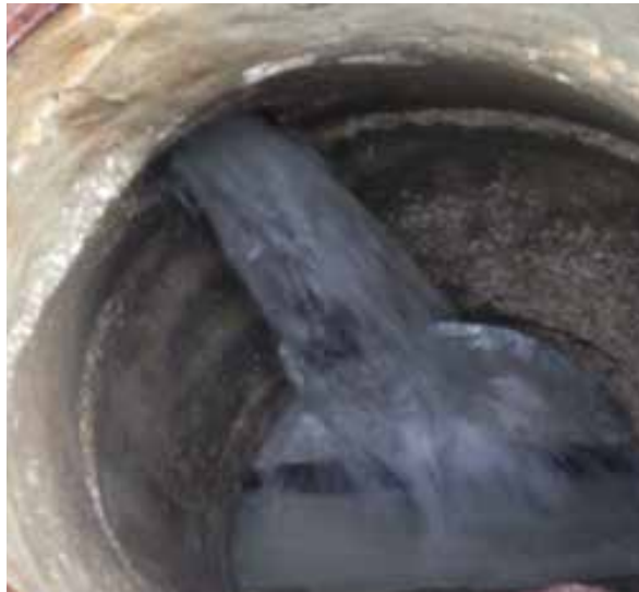
Figure 7-13 Intrusion of storm water in Sewerage Network through a manhole
