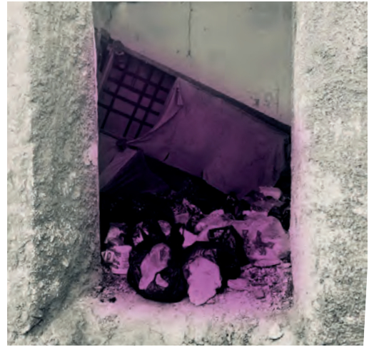
Health Hazardous Area
