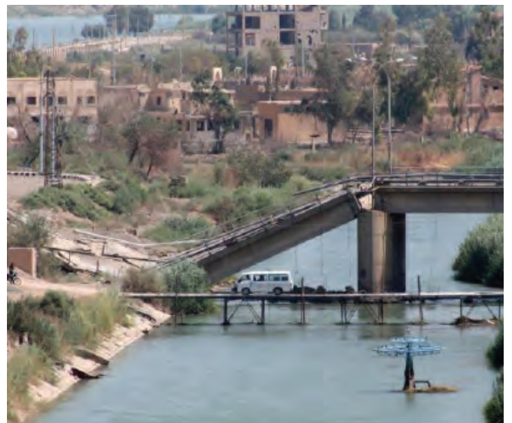
The damaged Suspension Bridge Deir Ez-Zour
