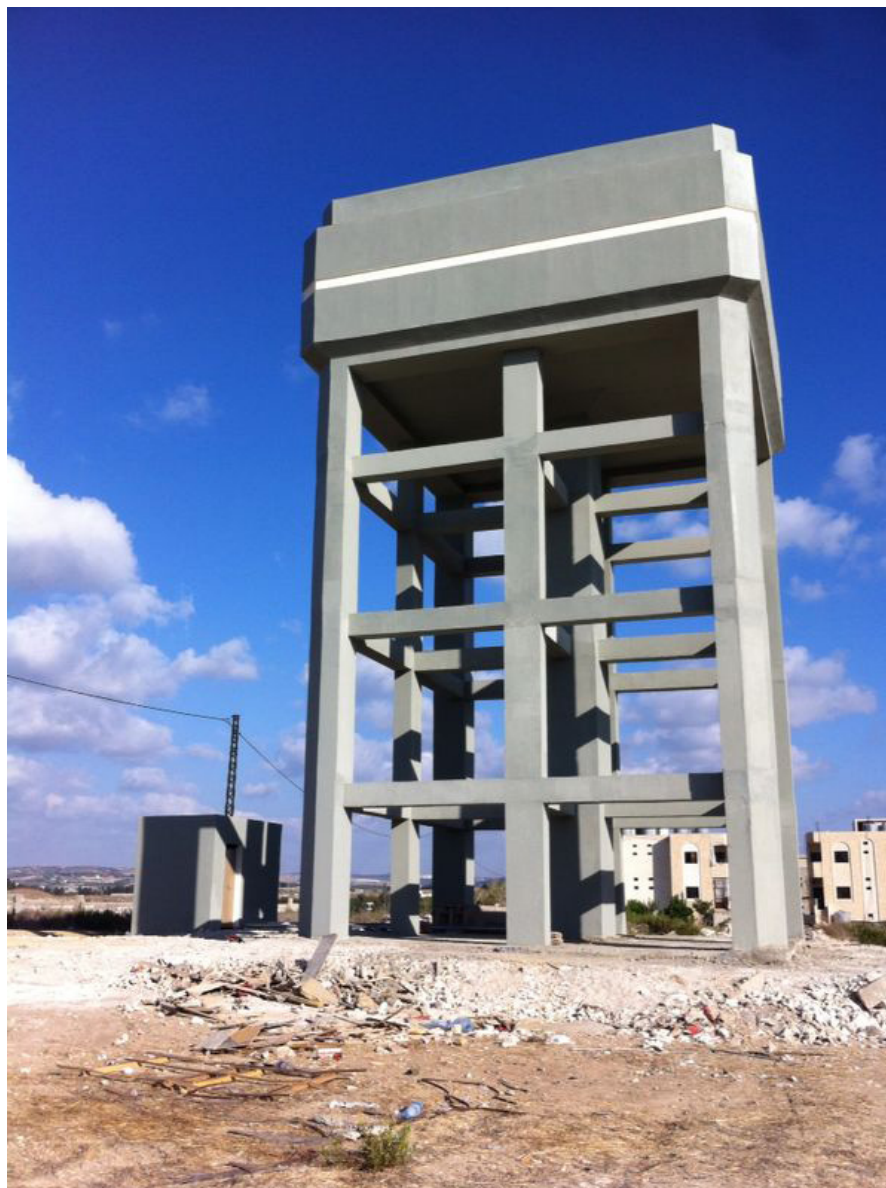
Water reservoir implemented in Ansarieh providing one of the basic needs
