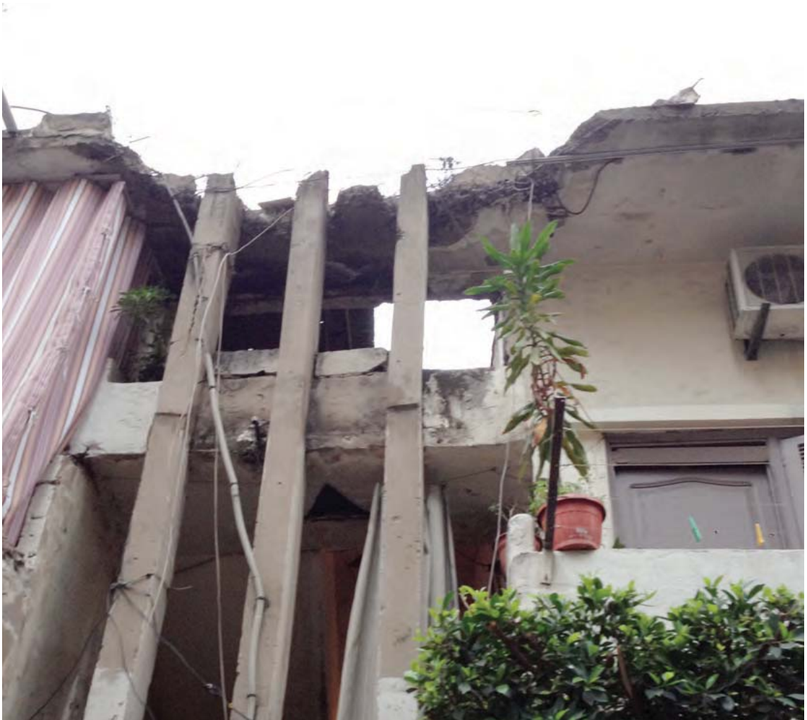
Picture 8: Dilapidated building in Naba'a - Beirut, Lebanon
