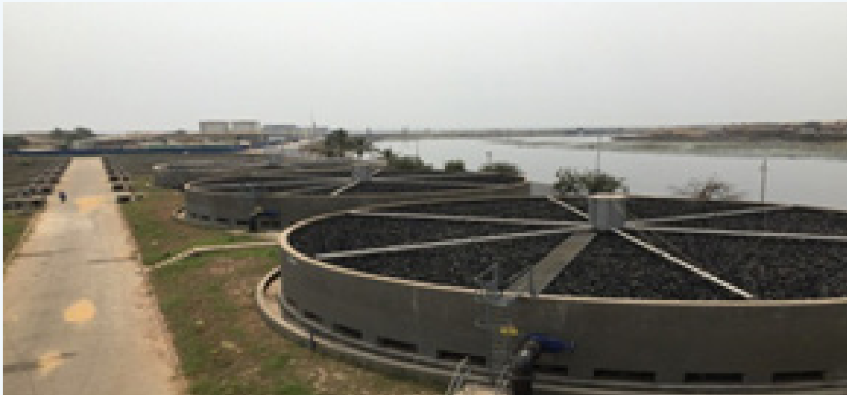
Figure 2.8 Mudor Sewage Plant and Sanitation Equipment
