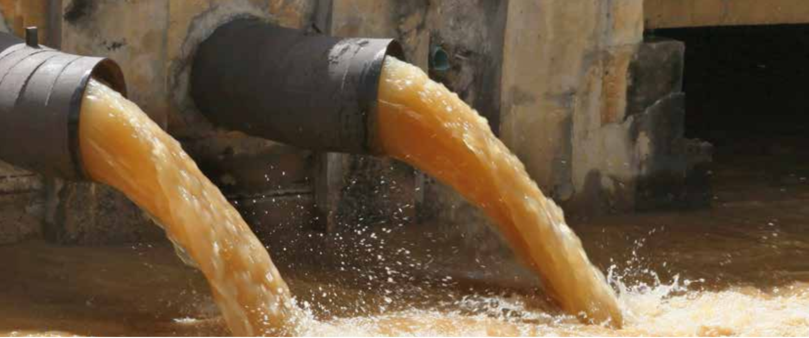
Water flowing at a wastewater treatment facility. Photo: Shutterstock
