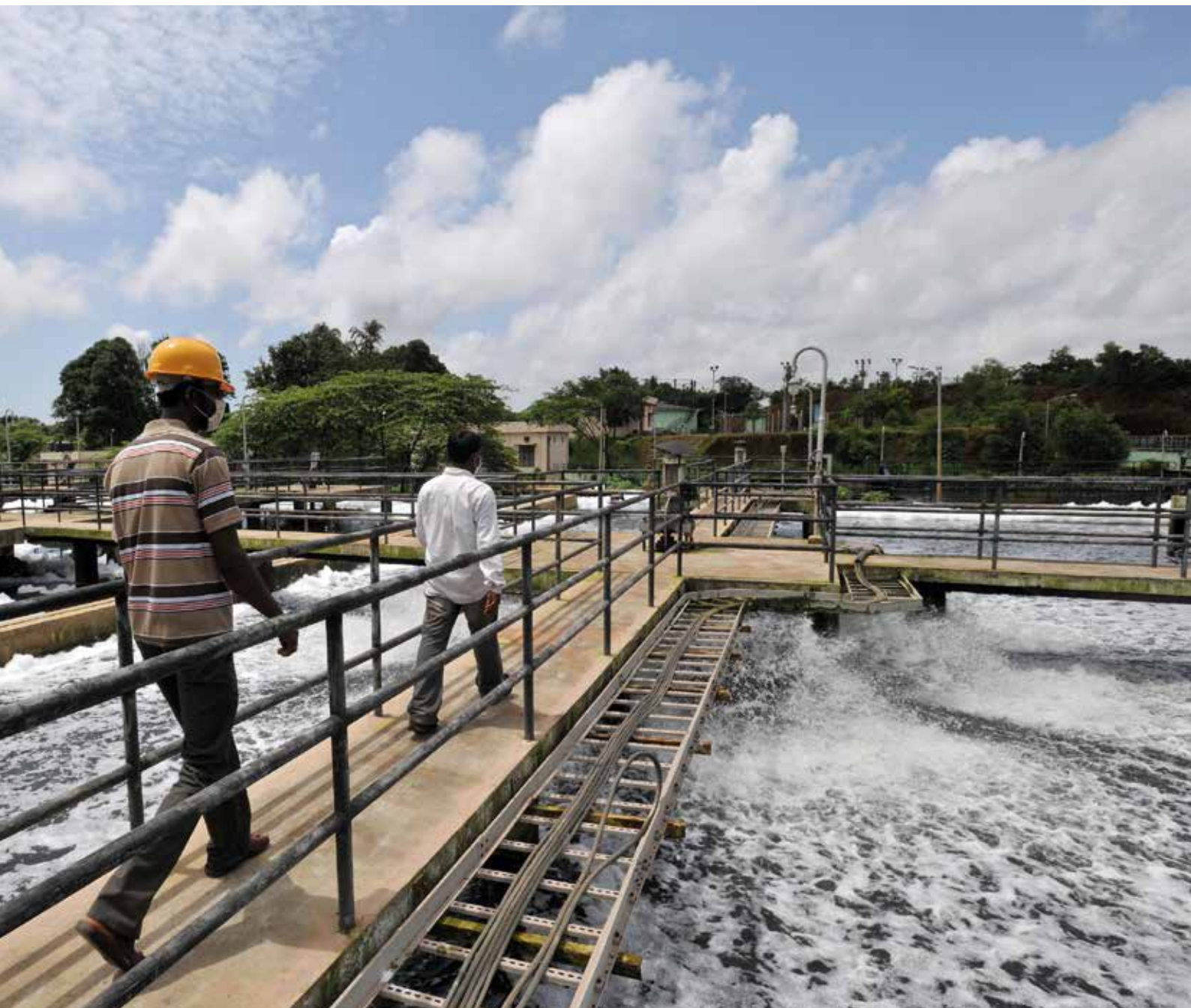
Sewage treatment plant in Kavoor, Mangalore, India. Photo: Asian Development Bank
