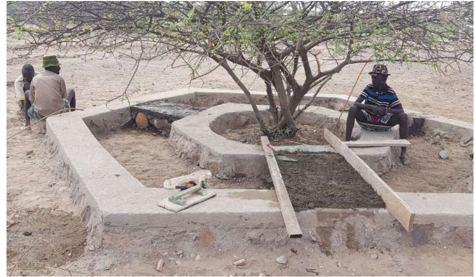
Beginning of construction process of local game area, using cement and soil
