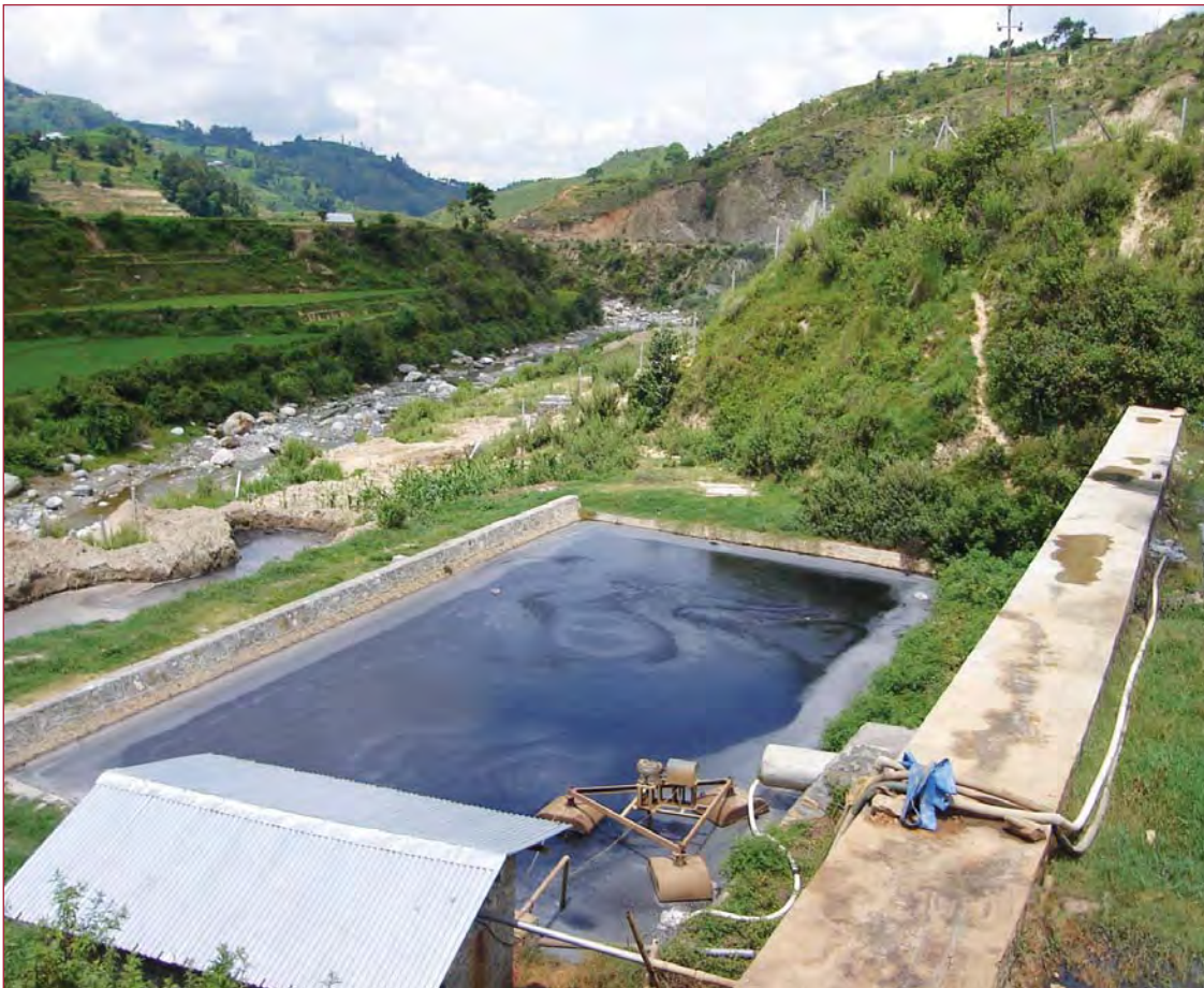
Leachate treatment systems form one of the key elements for upgrading landfill practices, Ghorahi, Nepal
