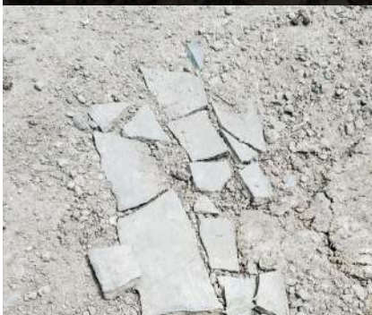
Presumed asbestos-containing cement products
