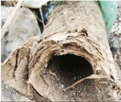
Presumed asbestos-containing paper mechanical insulation
