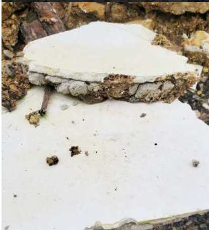
Presumed asbestos-containing plaster application
