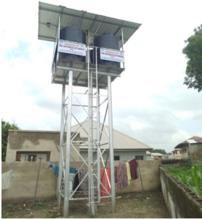
» Smart-Metered Solar Borehole in Niger State (Nigeria)
