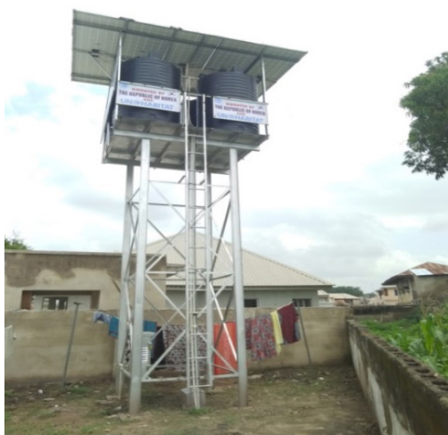
» Smart-Metered Solar Borehole in Niger State (Nigeria)
