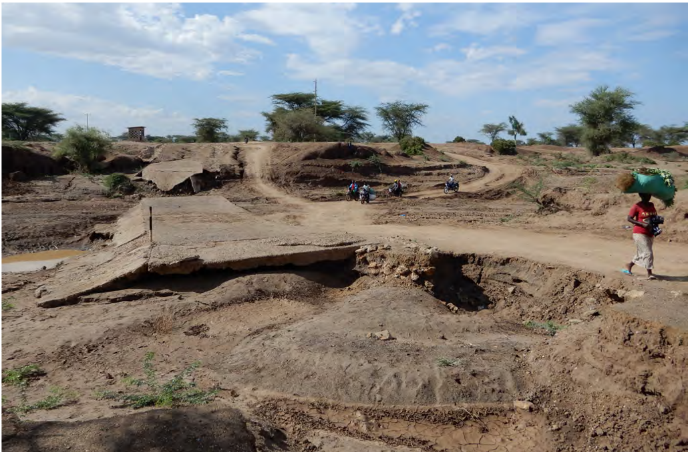
Fig. 33: Damaged Drift Near Fuji Primary School, Connecting Kakuma Camps 1 and 2 (UN-Habitat, 2023)
