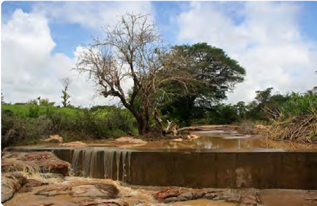
Figure 150 A Sand Storage Dam shortly after the first rains of the wet season (2005) 233
