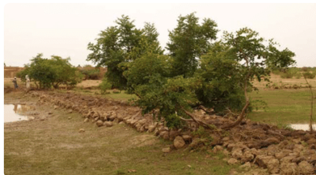
Figure 45 An example of a permeable rock dam (PRD) being used for Soil and Water Conservation (SWC) 66
