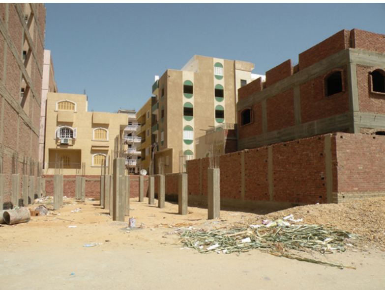
Figure 4.12 Formal private housing at various stages of completion on 600 m 2 plots, New Cairo, 2009.
