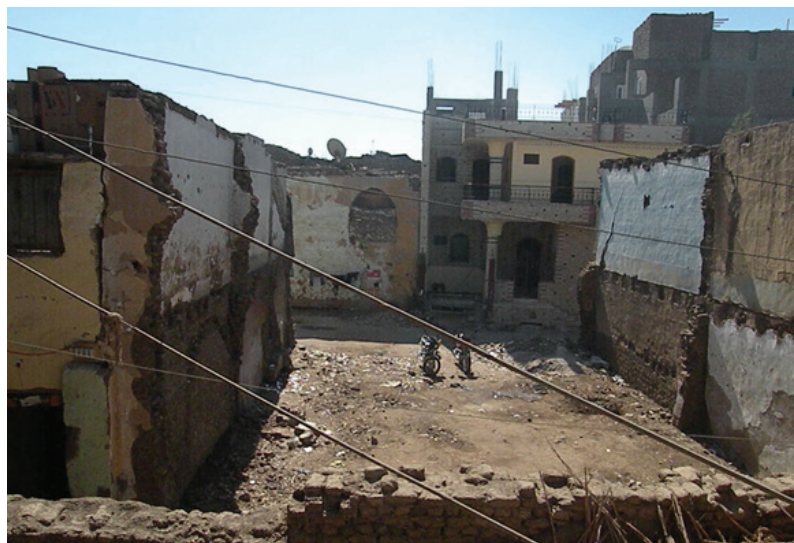
Figure 1.2 Remains of some of the few original mud brick houses in New Gurna, 2009. Photo by D. Sims
