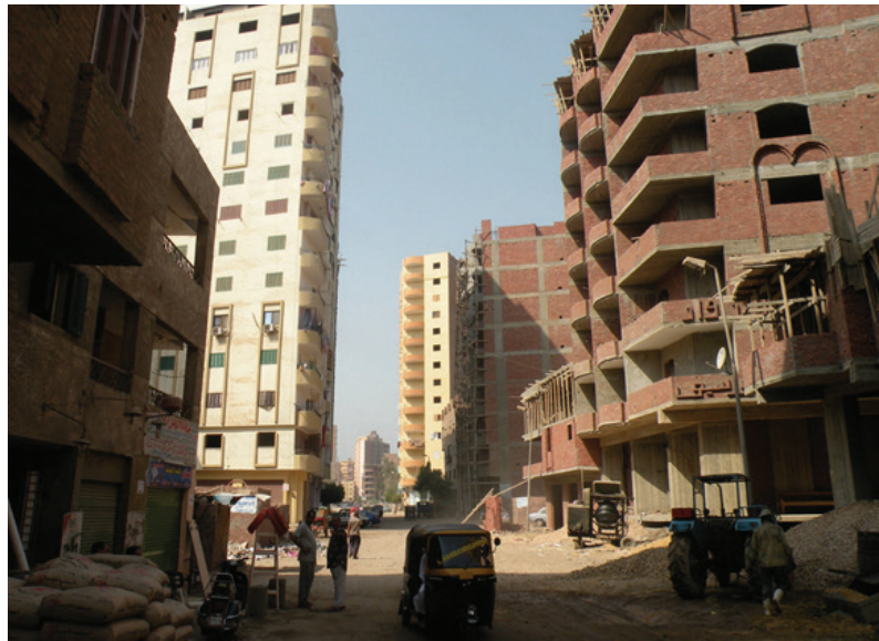
Figure 4.15 Informal one-off tower blocks under construction, Boulaq al-Dakrou, 2009. Photo by D. Sims.
