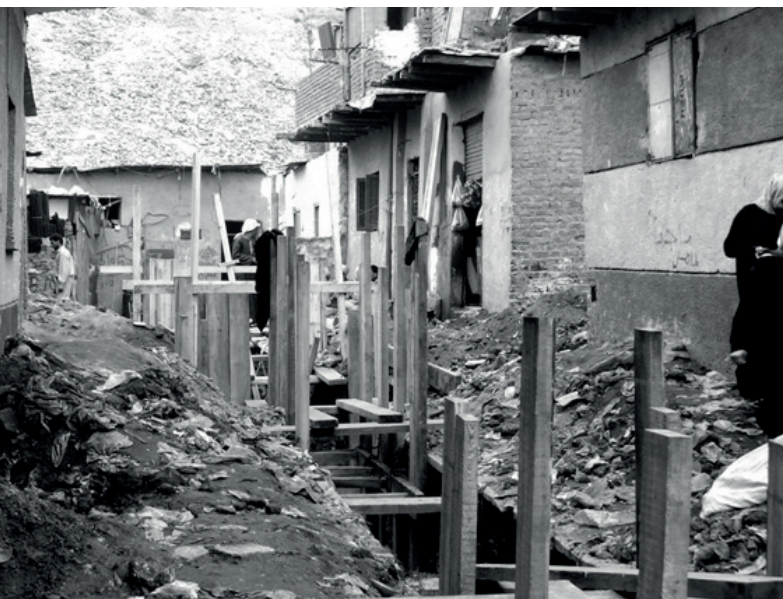
Figure 10.1 Installing sewers in a mature informal settlement on State land (Ezbet Bekhit, Manshiet Nasser), financed by KfW, 2002. Photo by D. Sims
