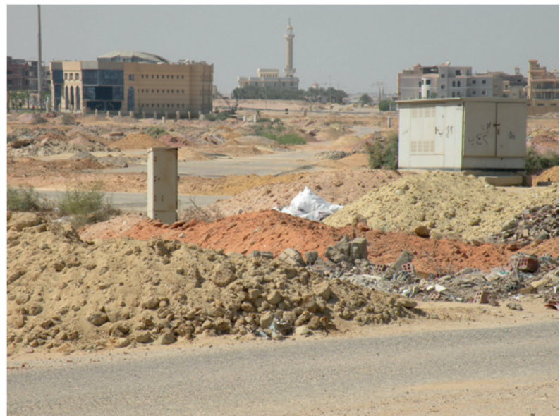
Figure 10.5 Electrical transformer and distribution box, New Cairo subdivision, 2009. Photo by D. Sims
