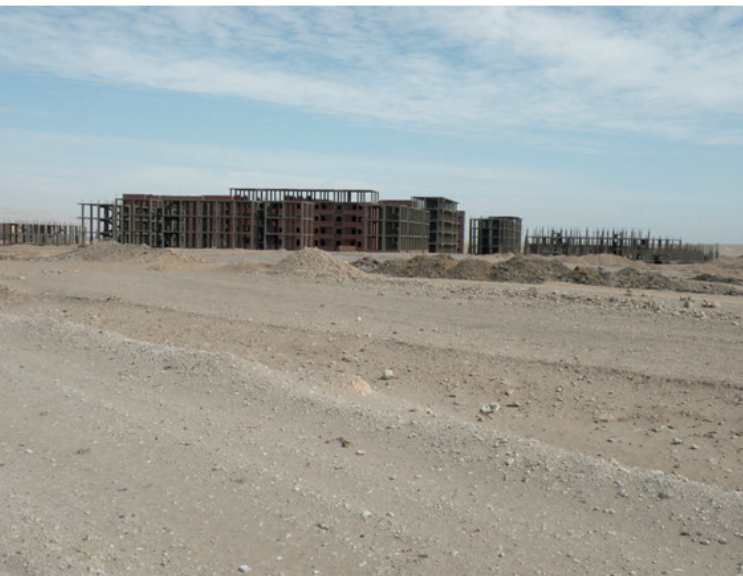
Figure 7.6 Governorate public housing under construction on remote desert site in unplanned rural area, Al Tarif, Luxor, 2015. Photo by D. Sims.
