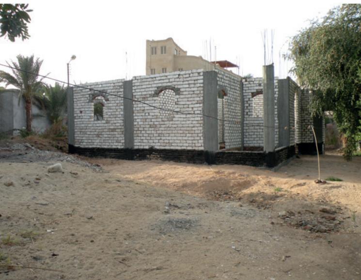
Figure 11.8 Use of soft limestone block as a cheaper alternative to red brick for wall infill. Al Bairat, Luxor Governorate, 2015. Photo by D. Sims.
