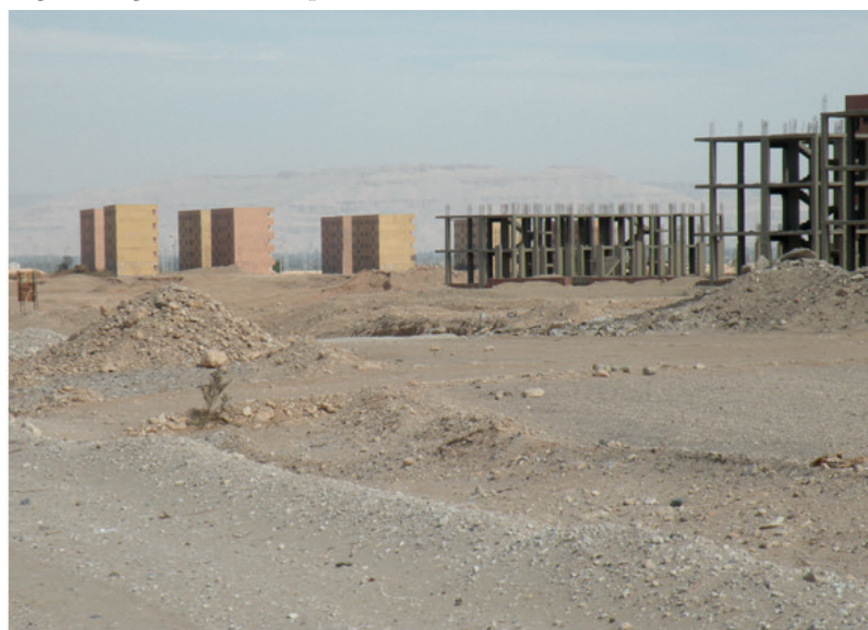
Figure 11.2 Public housing blocks under construction, Al Tarif, Luxor Governorate, April 2015. Photo by D. Sims
