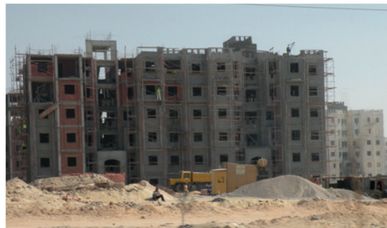
Figure 11.1 Cooperative housing blocks under construction, Sixth of October, 2010. Photo by D. Sims
