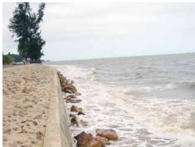
Sea wall along Maputo coastline ©UN-HABITAT/B.Oballa
