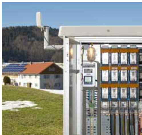
A smart grid at work in Wildpoldsried, Allgäu, Germany © Siemens
