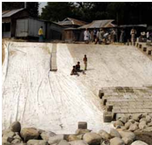
Reinforced river embankment along the Brahmaputra River in Dhaka, Bangladesh © Leila Mead/IISD
